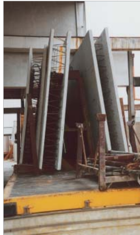
Finished double walls on the way to the construction site. After installation they will be filled with site concrete
