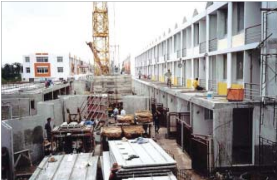
The same system, but a completely different building: this multi-story building – also in Thailand – is planned for housing and businesses
