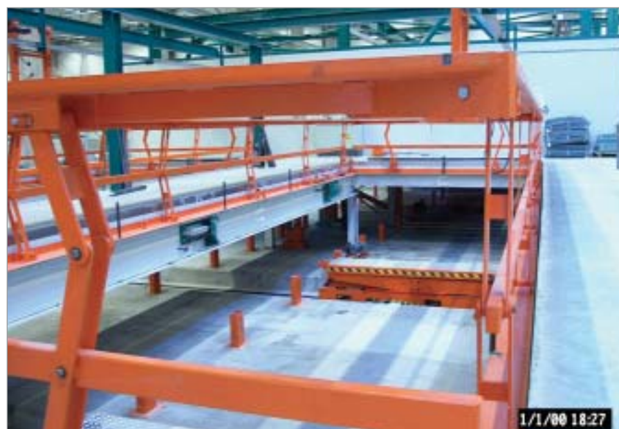
Bottom: Elevating platform truck at transport level. Top: Processing level 02
