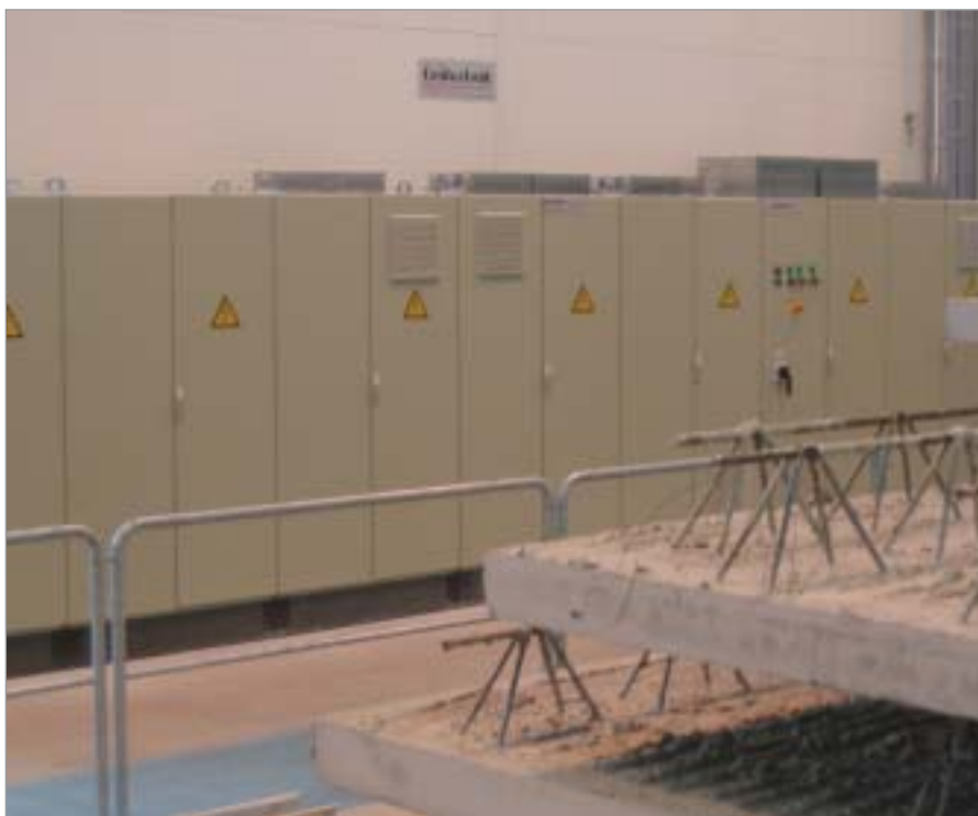
Circulation switch cabinet
