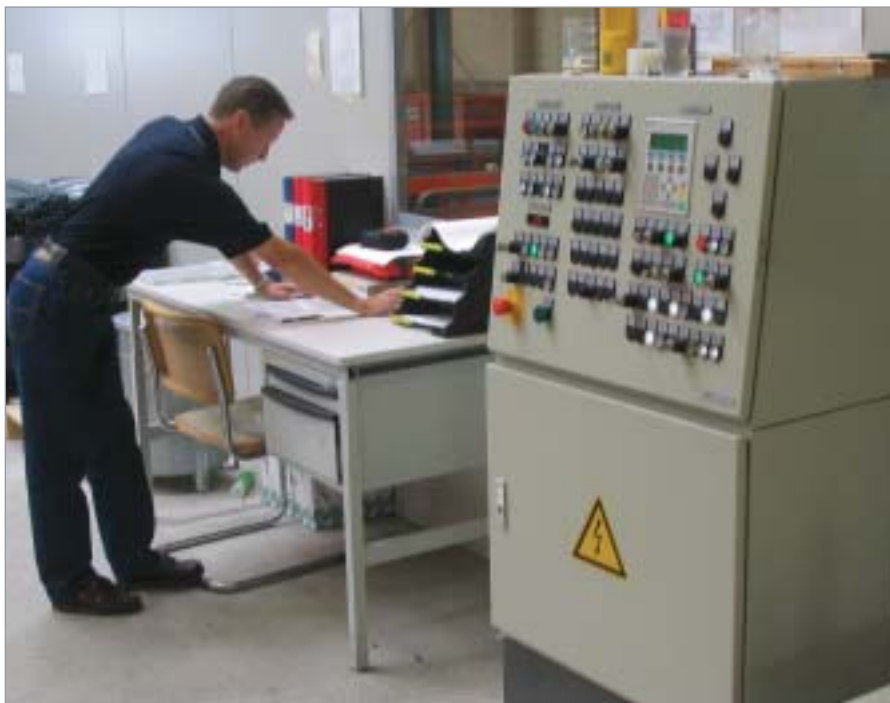
Circulation control station
