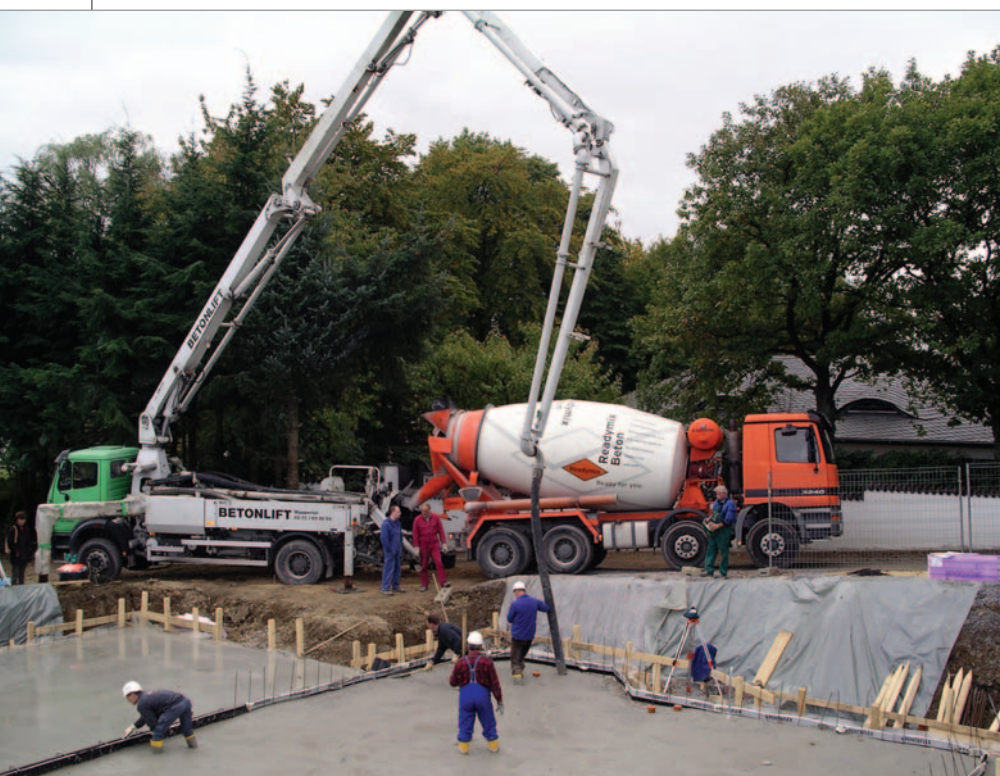
Base plate from Aaton steel fibre - preparations and pouring the concrete for the base plate were completed in only two days
