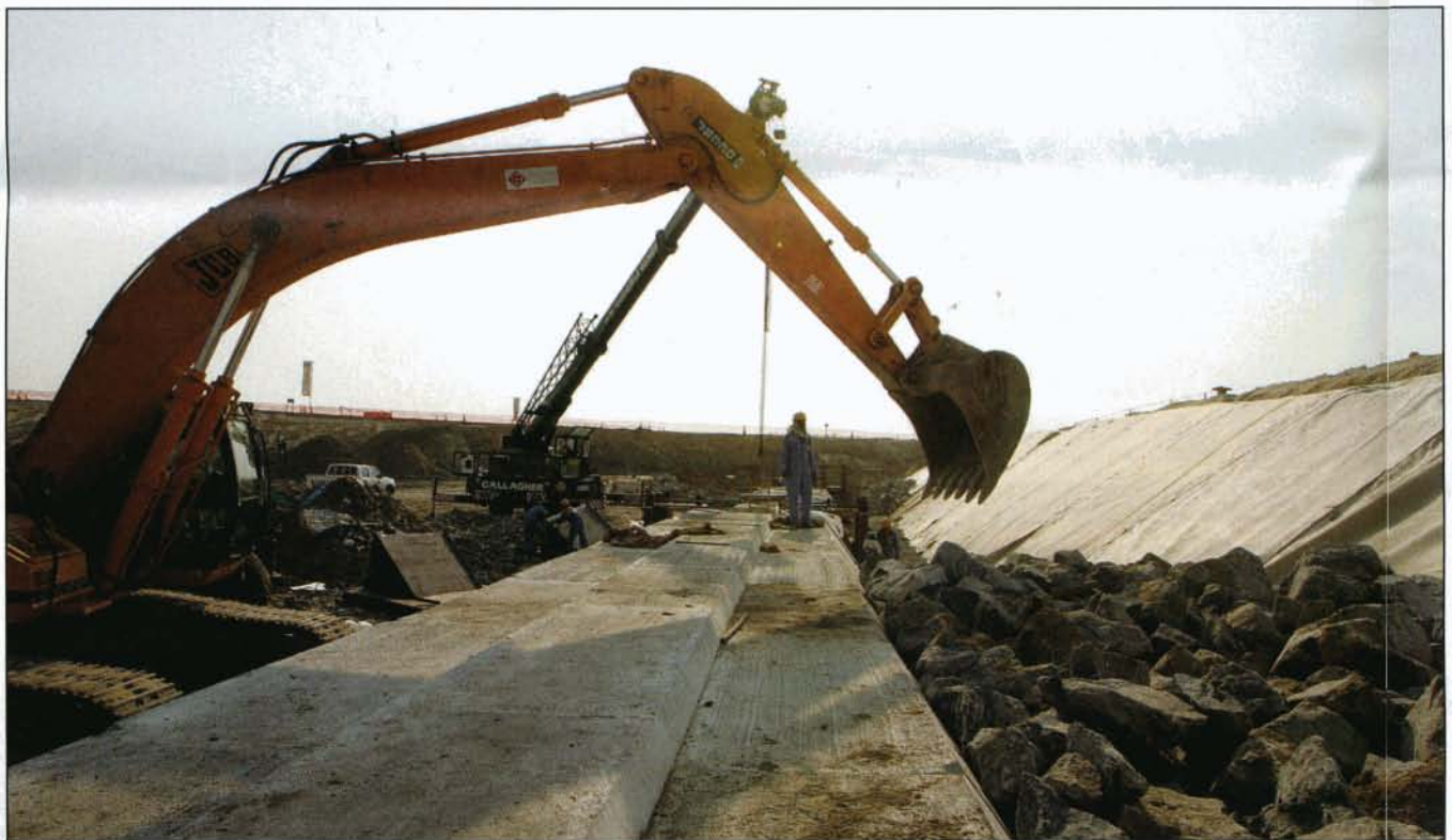
Rock hard: The Quay wall on the Creek extension project is being constructed using precast mass concrete gravity blocks with crush rock foundations.
